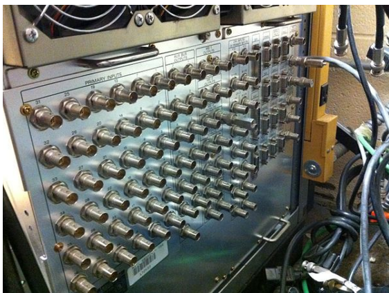
Rear of a video switcher with an array of BNC connectors
