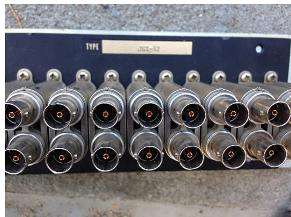
Rear view of a patch panel with BNC jacks in close proximity. [11]
